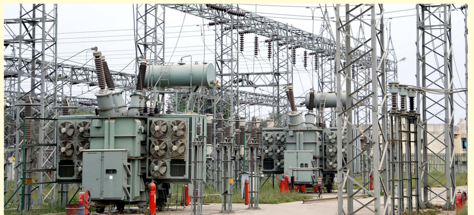
100 MVA, 220/132/11 KV Auto Transformer
