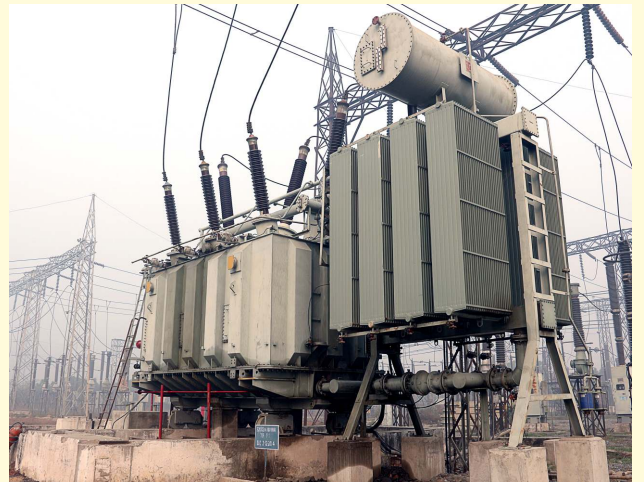
160 MVA, 220/132/11 KV, Auto Transformer
