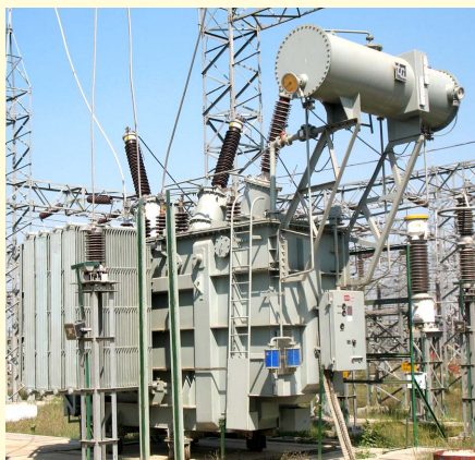
40 MVA, 132/33 KV Power Transformer
