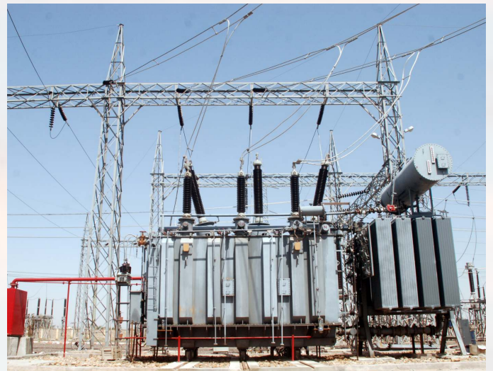
160 MVA, 220/132/11 KV, Auto Transformer
