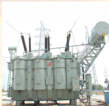
100 MVA, 220/132/11 KV Auto Transformer
