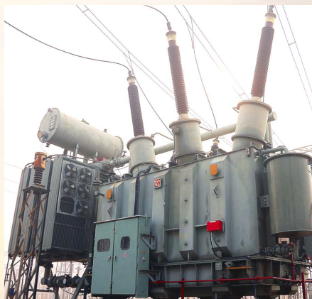
100 MVA, 220/132 KV Power Transformer
