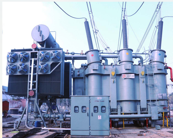
100 MVA, 220/33/11 KV Power Transformer
