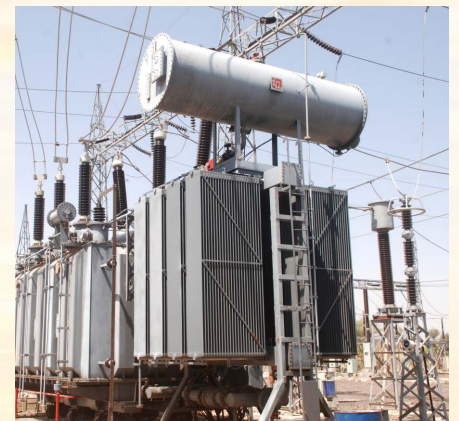
160 MVA, 220/132/11 KV, Auto Transformer
